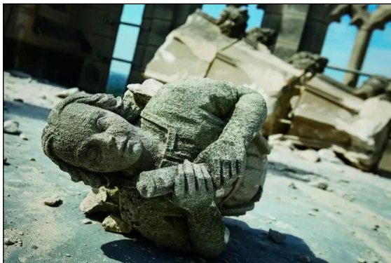
An angel carved of stone lies damaged on the Washington National Cathedral tower following the 2011 Virginia Earthquake that caused extensive damage to the cathedral (Photo: Washington National Cathedral).
